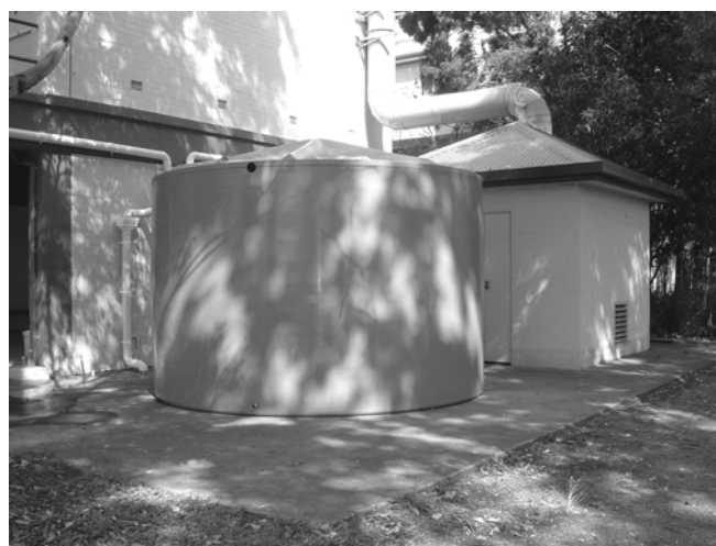
One of our 22,000L water tanks at the end of H Block
